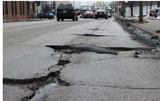
Roads in need of repairs
